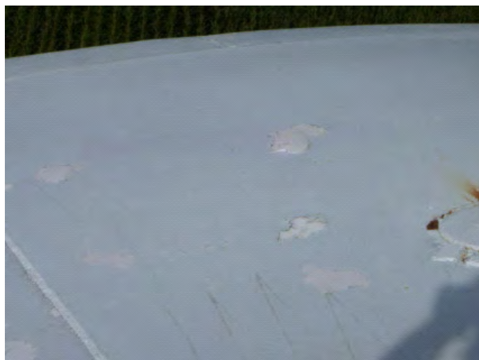
Top coat delamination on roof
