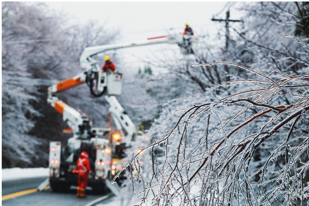
Image: Utility crew responds to infrastructure affected by winter weather (Getty)
