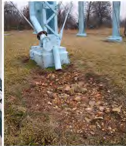
PHOTOGRAPH #8 & #9 TAKEN BY: Clinton Finn ENTITY: Neosho PWS PERMIT: MO5010560 LOCATION: Camp Crowder DESCRIPTION: NE Elevated Crowder Tank and Overflow Pipe DATE TAKEN: January 26, 2021 PROGRAM: Public Drinking Water Branch
