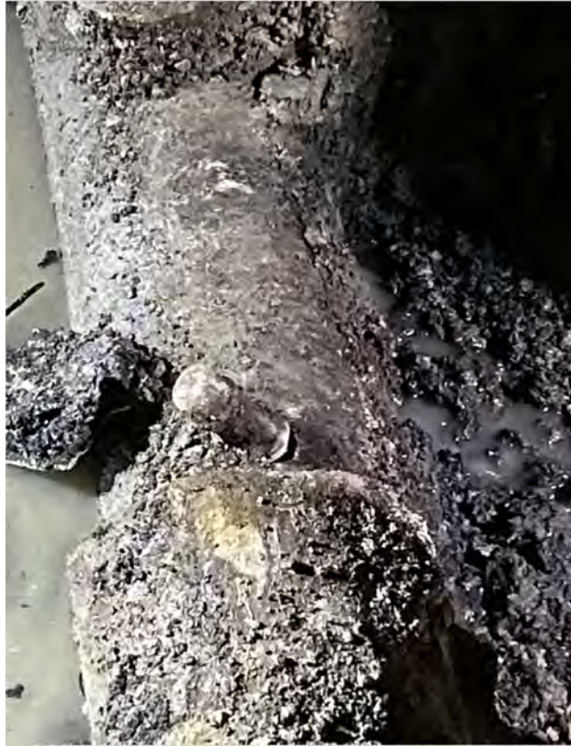
Figure 2: Damaged Fitting on Main (Source: Spire Response to Staff Data Request 0001.3A)
