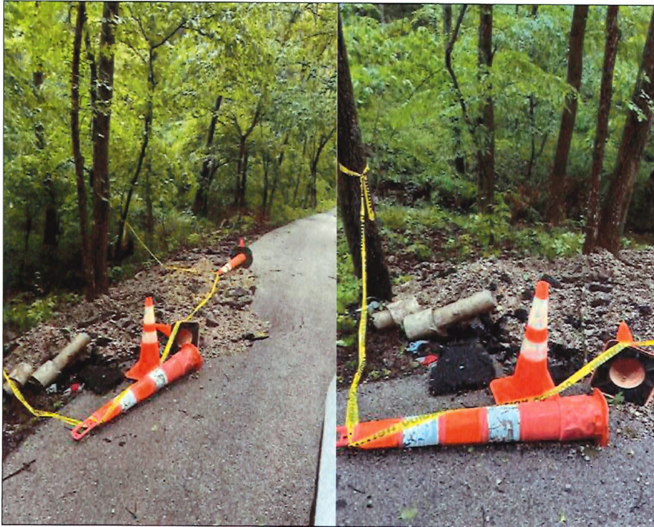
Photo 5 — Close-up taken May 19, 2026 at 6:16:57 AM. AC pipe sections clearly visible alongside collapsed cones and caution tape. Gravel fill spread across road surface. Wooded drainage corridor visible in background — direct pathway to [REDACTED] watershed.
