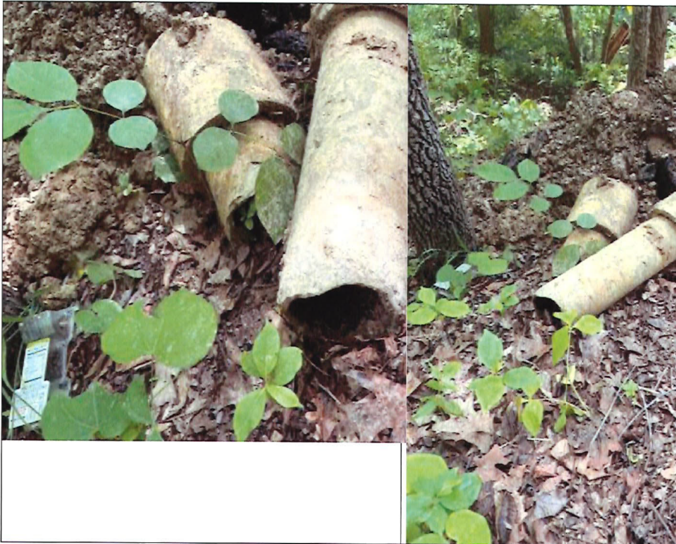
Photo 1 — Close-up of broken AC pipe sections. Multiple pieces visible with fractured ends exposing asbestos cement material. Taken May 17, 2026, 12:09 PM.
