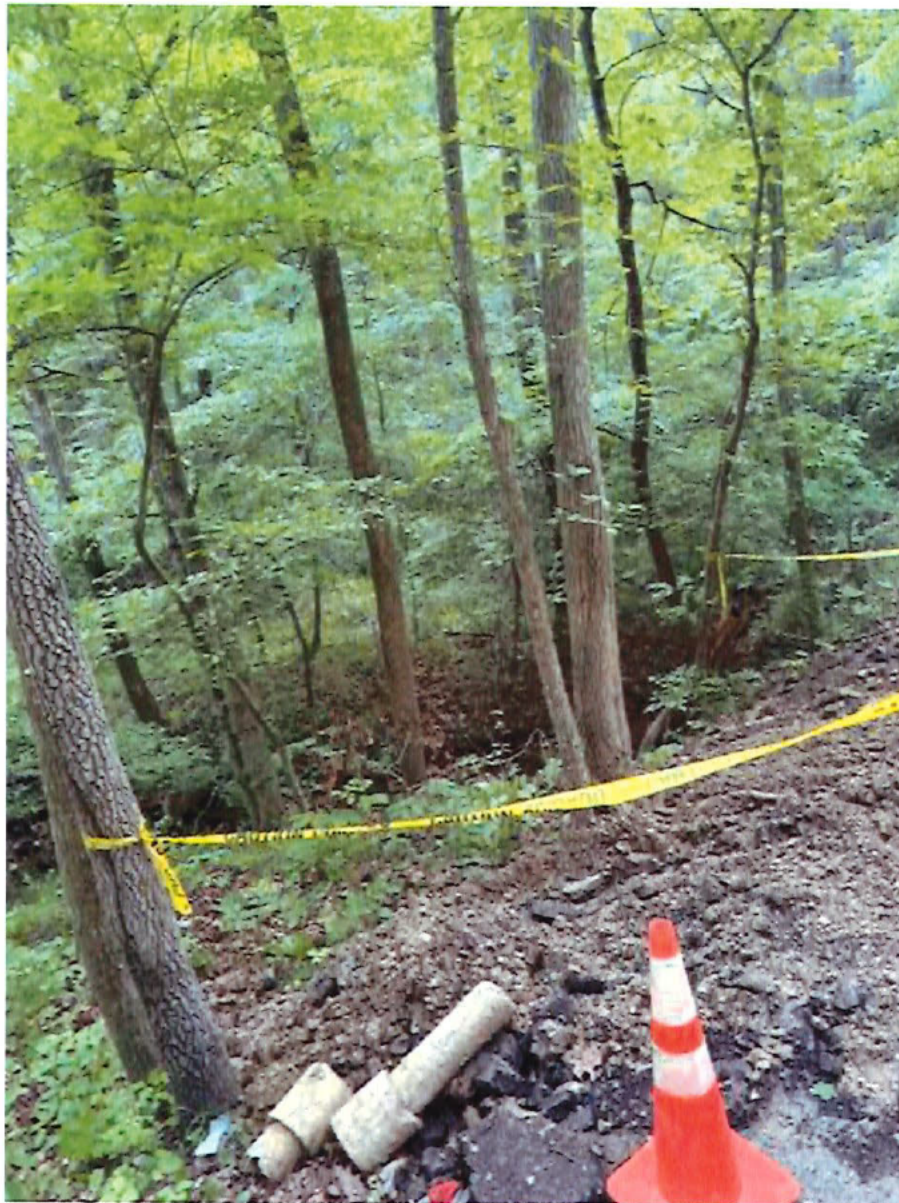
Photo 3 — Site overview taken May 18, 2026 at 6:25 AM showing AC pipe sections still in place. Yellow caution tape visible strung between trees. Road surface wet — active rainfall conditions. Site drains directly into wooded area at left. Traffic cone at lower right.
