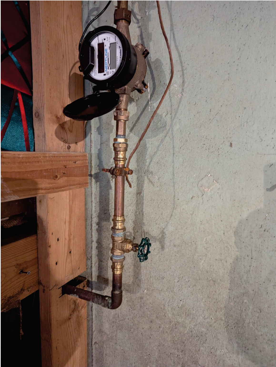
My Personal photo on March 4th, 2026 of the defective valve
