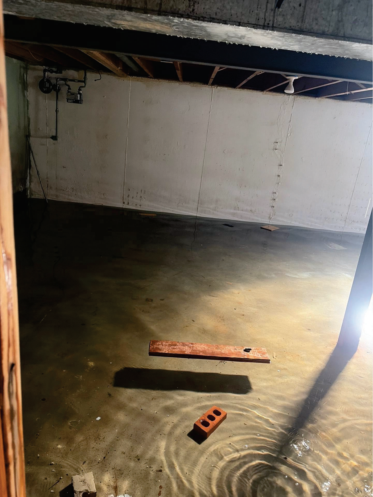
Water Flood incident 2/26/2026
