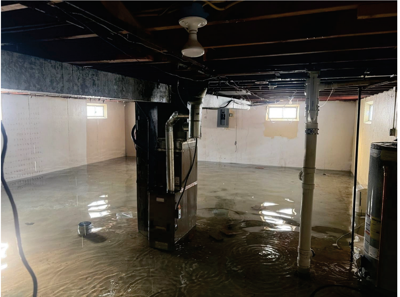
Hvac and water tank under water
