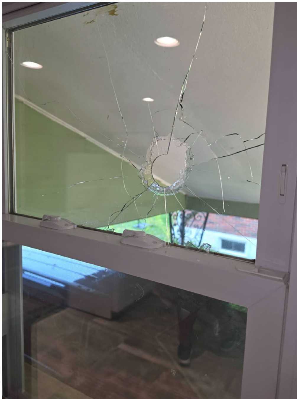
New: Vandalized new window.
