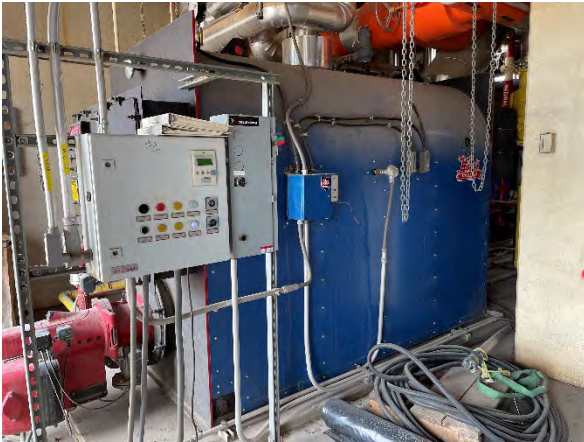
Photo #: 4 Taken By: Christina Kerr Entity: Blue River WWTP Permit: 095-0039 Location: 7300 Hawthorne Road, Kansas City Description: 2016 Digester gas boiler 6.3 MMBtu/hr. Date Taken: July 25, 2023 Media: KCRO Air Unit
