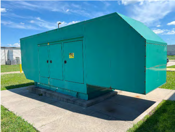
Photo 7 Taken By: Christina Kerr Entity: Blue River Wastewater Treatment Plant Facility ID: 095-0039 Location: 7300 Hawthorne Road, Kansas City Description: 2013 Cummins natural gas emergency generator set, model 35OGFEB. Date Taken: July 2, 2025 Media: Air Pollution Control
