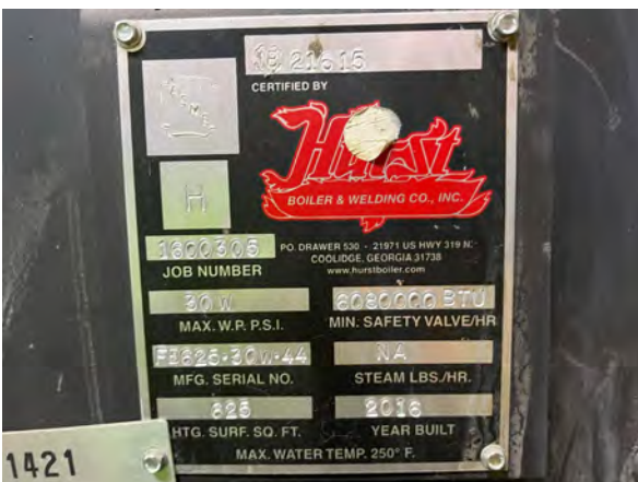
Photo 3 Taken By: Christina Kerr Entity: Blue River Wastewater Treatment Plant Facility ID: 095-0039 Location: 7300 Hawthorne Road, Kansas City Description: Data plate for digester gas boiler 1. Date Taken: July 2, 2025 Media: Air Pollution Control
