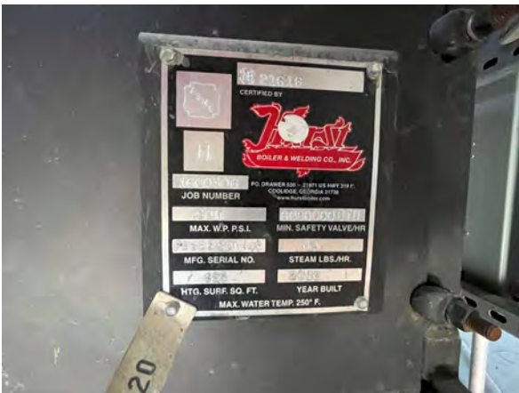
Photo 5 Taken By: Christina Kerr Entity: Blue River Wastewater Treatment Plant Facility ID: 095-0039 Location: 7300 Hawthorne Road, Kansas City Description: Data plate for digester gas boiler 2. Date Taken: July 2, 2025 Media: Air Pollution Control
