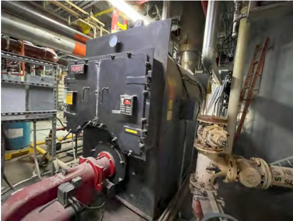
Photo 4 Taken By: Christina Kerr Entity: Blue River Wastewater Treatment Plant Facility ID: 095-0039 Location: 7300 Hawthorne Road, Kansas City Description: 2016 digester gas boiler 2. Date Taken: July 2, 2025 Media: Air Pollution Control
