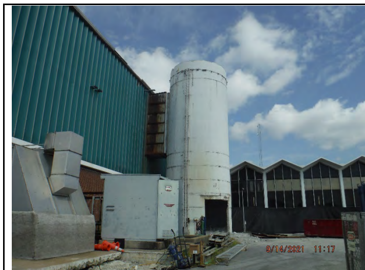
Photograph: 1 Taken By : Daniel Simmons Date Taken: September 14, 2021 Program: KCRO, Air Pollution Control Unit Entity: Blue River Wastewater Treatment Plant Facility ID: 095-0039 Location: 7300 Hawthorne Rd, Kansas City Description: Dismantled incinerator stack
