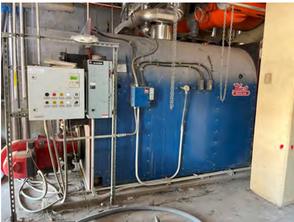
Photo 2 Taken By: Christina Kerr Entity: Blue River Wastewater Treatment Plant Facility ID: 095-0039 Location: 7300 Hawthorne Road, Kansas City Description: 2016 digester gas boiler 1. Date Taken: July 2, 2025 Media: Air Pollution Control
