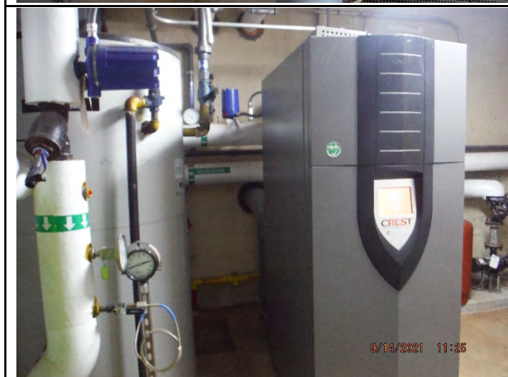
Photograph: 3 Taken By: Daniel Simmons Date Taken: September 14, 2021 Program: KCRO, Air Pollution Control Unit Entity: Blue River Wastewater Treatment Plant Facility ID: 095-0039 Location: 7300 Hawthorne Rd, Kansas City Description: Odor control system
