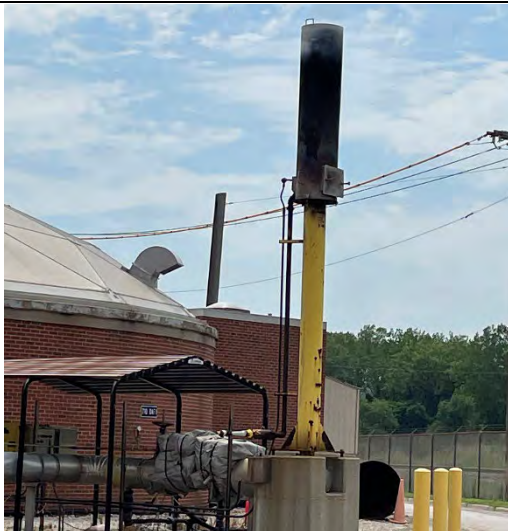
Photo #: 6 Taken By: Christina Kerr Entity: Blue River WWTP Permit: 095-0039 Location: 7300 Hawthorne Road, Kansas City Description: Sludge Digester Flare Date Taken: July 25, 2023 Media: KCRO Air Unit
