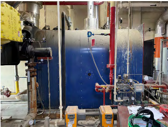
Photo #: 5 Taken By: Christina Kerr Entity: Blue River WWTP Permit: 095-0039 Location: 7300 Hawthorne Road, Kansas City Description: 2016 Digester gas boiler 6.3 MMBtu/hr. Date Taken: July 25, 2023 Media: KCRO Air Unit
