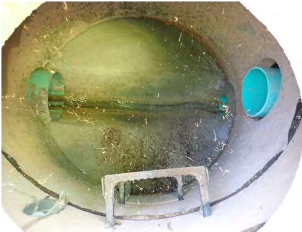
Photo: 2 Taken By: Denise Eagan Entity: Kansas City Permit: MO0024911 Location: 39.053480, -94.541017 Description: Viewing inside the new manhole which no longer has an overflow structure. Date Taken: June 10, 2025 Media: CW
