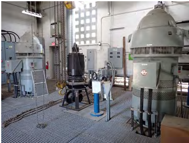
Photo: 11 Taken By: Denise Eagan Entity: Kansas City Permit: MO0024911 Location: 39.076999, -94.602132 Description: Viewing the two stormwater pumps and one sanitary pump. Date Taken: June 10, 2025 Media: CW
