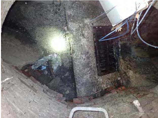
Photo: 22 Taken By: Denise Eagan Entity: Kansas City Permit: MO0024911 Location: 7300 Hawthorne Rd Description: Viewing inside diversion structure 115 with flow meter. Date Taken: June 10, 2025 Media: CW
