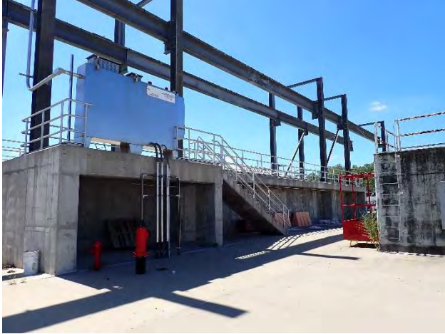
Photo: 7 Taken By: Denise Eagan Entity: Kansas City Permit: MO0024911 Location: 39.085257, -94.606802 Description: Viewing the gravity feed into the pump station with diversion on the right. Date Taken: June 10, 2025 Media: CW
