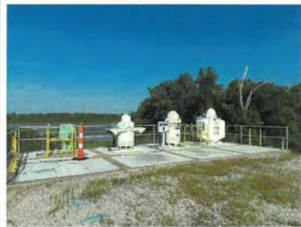
INTAKE PUMP HOUSE
