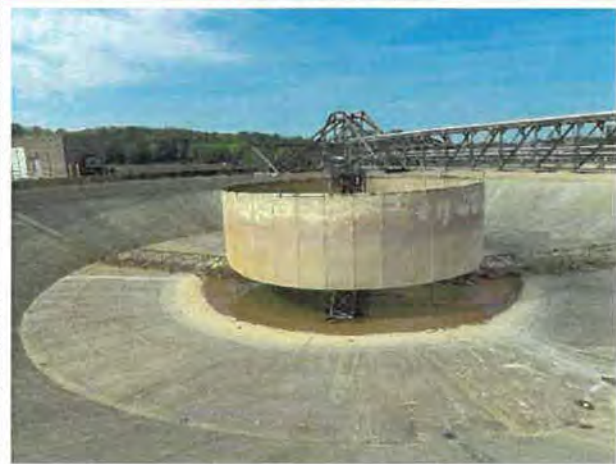
VIEW OF AERATOR
