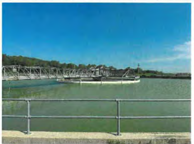
VIEW OF AERATOR
