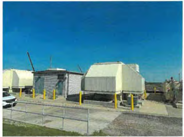
VIEW OF ON-SITE GENERATORS
