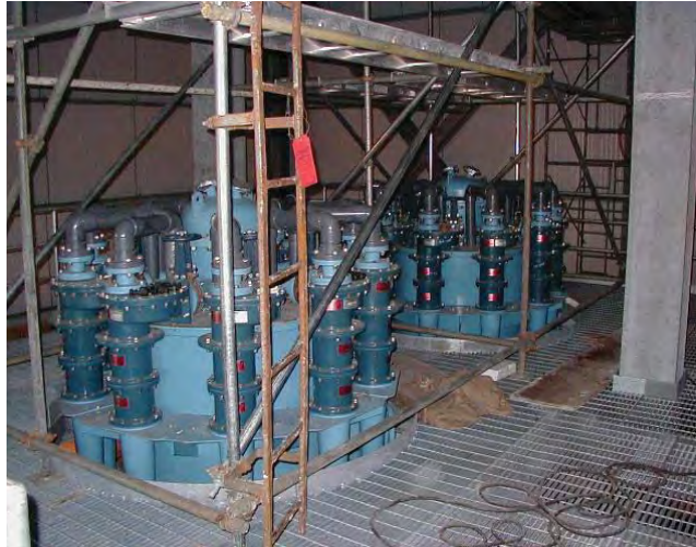
Figure 2-7 – Hydrocyclones for Primary Gypsum Dewatering
