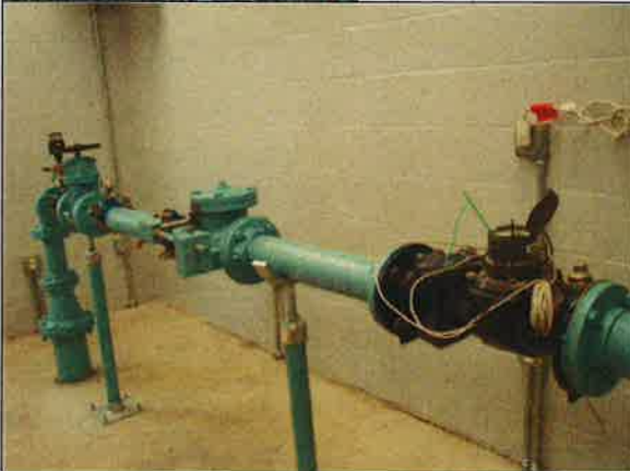
Photo #:012 Date Taken: 10/26/2016 By: Michelle Oglesby Program: PDWB File: Crawford County Location: Indian Hills Utilities Operating Co. Inc. Description: Well #3 - Piping
