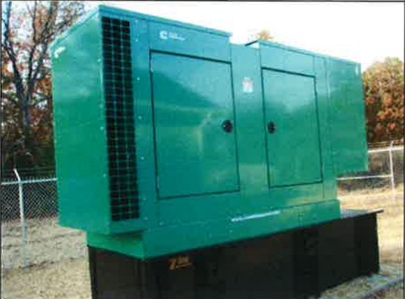
Photo #:008 Date Taken: 10/26/2016 By: Michelle Oglesby Program: PDWB File: Crawford County Location: Indian Hills Utilities Operating Co. Inc. Description: Well #1 – Generator
