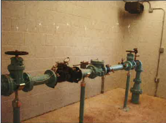
Photo #:002 Date Taken: 10/26/2016 By: Michelle Oglesby Program: PDWB File: Crawford County Location: Indian Hills Utilities Operating Co. Inc. Description: Well #1 - Piping
