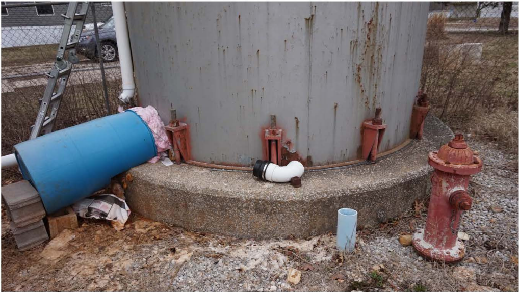
Willows Drinking Water Connection through 55-gallon drum stuffed with insulation on Cinder Blocks
