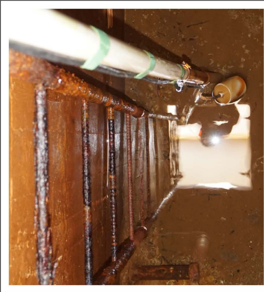
Inside of Roy-L's Drinking Water Tank Covered with Rust Sludge
