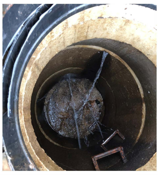
Infiltration and Inflow running into a Roy-L Manhole
