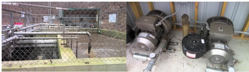
New aeration piping, blowers, and valving
