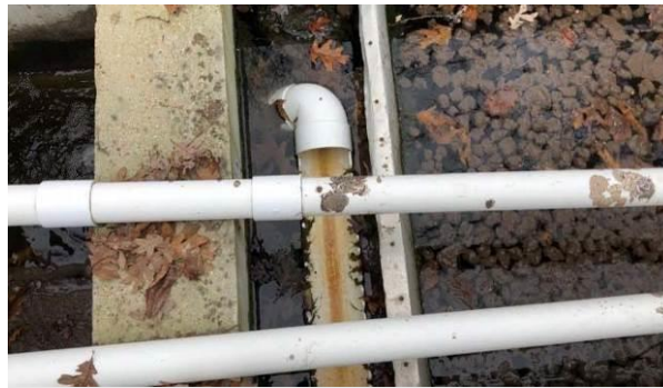
9 10 Sludge floating in clarifier basin, cobbled together PVC piping
