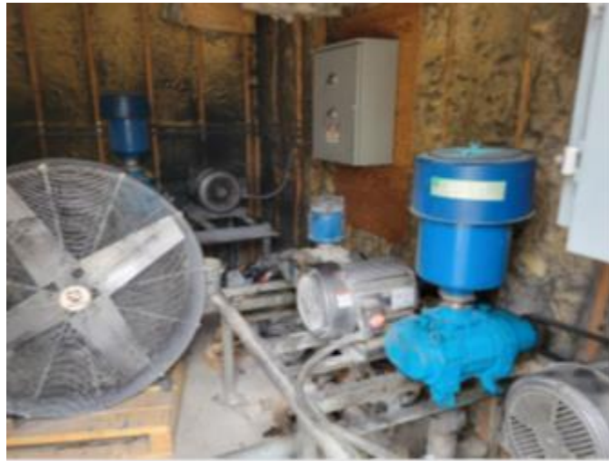
11 Poor condition of blower building interior, also visible electrical and control system with no ability to connect 12 emergency power source. 13 14
