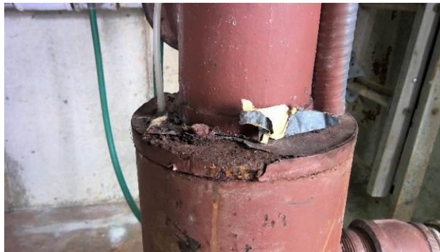
Rusting on well head at Cedar Green Well house.
