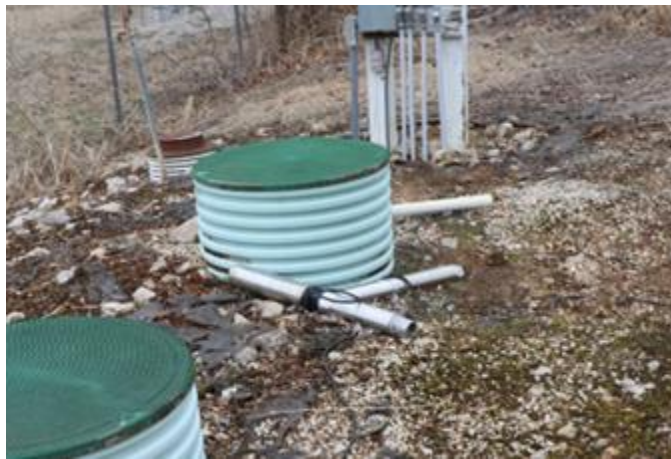
11 12 Pile of burnt-out submersible pumps near influent septic tank
