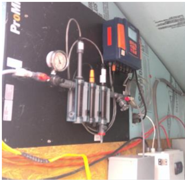
Chlorine Analyzer system
