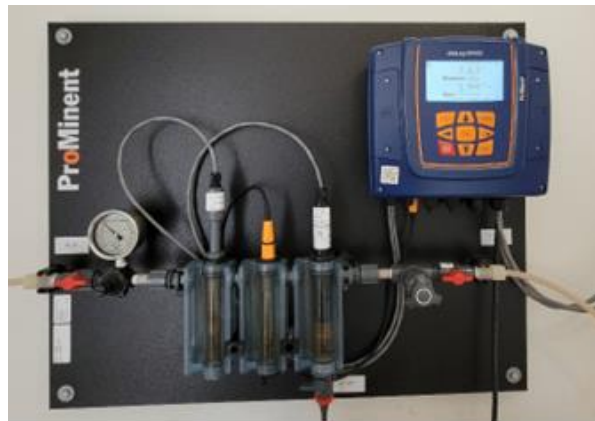
13 14 Chlorine Analyzer at Terre du Lac drinking water system 15
