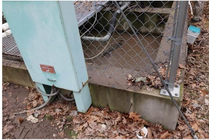
3 4 5 Completely full and overflowing digester at Chelsea Rose
