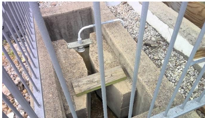
7 8 Ultrasonic Flow Meter at Cedar Green
