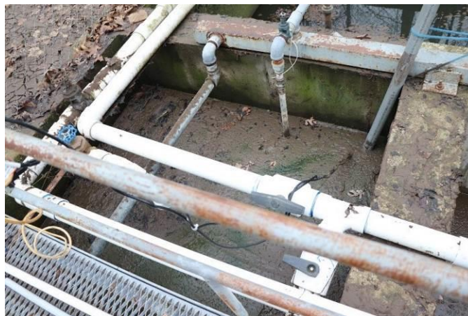
Overfilled sludge digester
