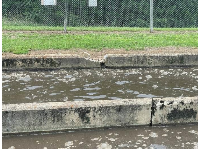
Examples of damaged concrete in oxidation ditch track
