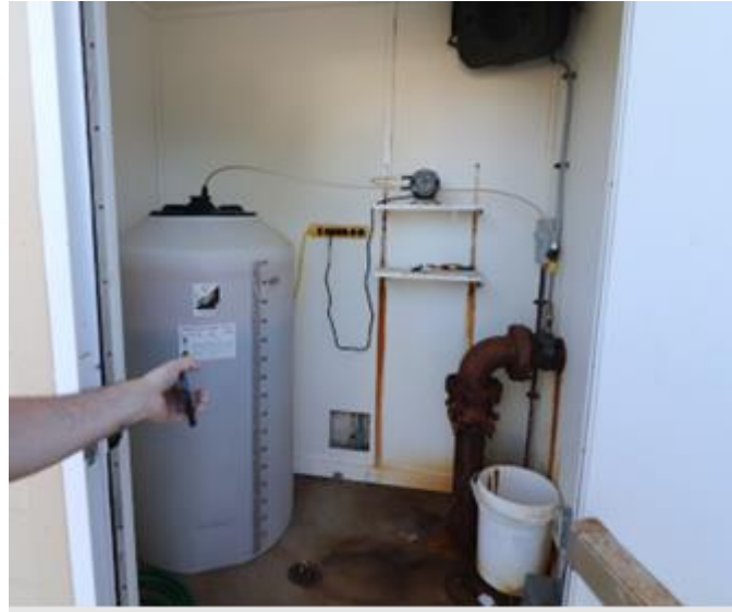
Well #4 disinfection room with steel rusting
