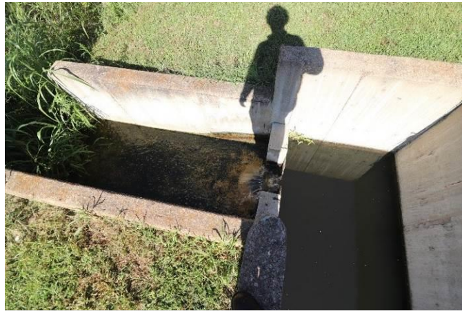
12 13 No dechlorination installed at end of contact chamber
