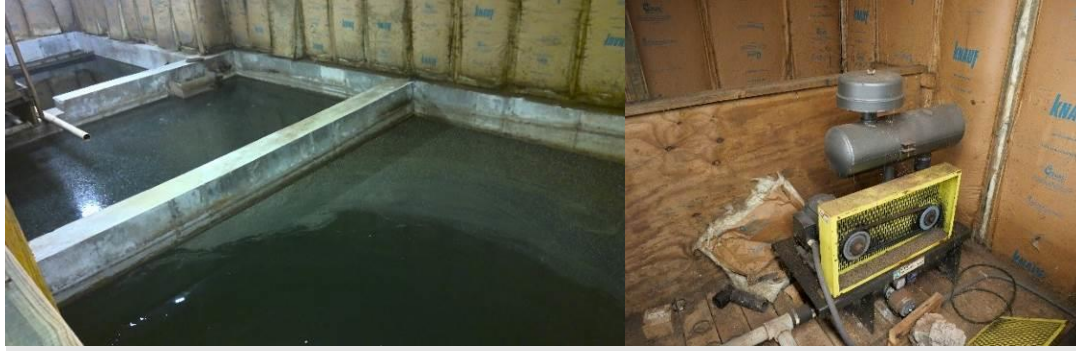
No functioning aeration present at Cedar Green and single failed blower
