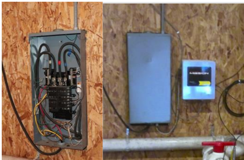
12 13 Damaged power panel, exposed wiring at Cedar Glen. Panel repaired and remote monitoring installed. 14
