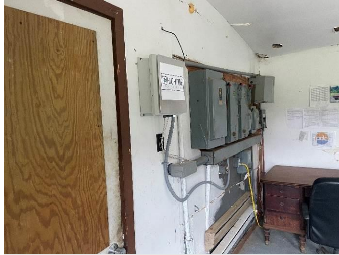
Remote monitoring equipment in Oxidation Ditch control room
