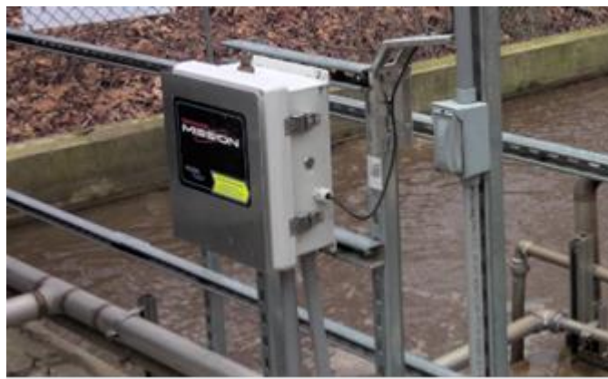
Newly installed remote monitoring system
