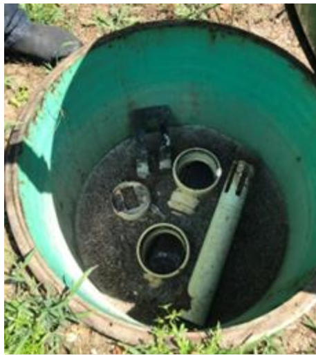
8 9 Damaged tablet chlorinator at Fox Run
