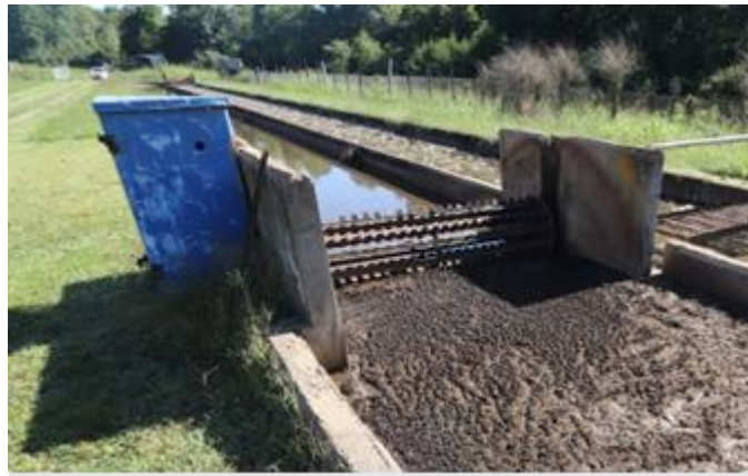
Failed brush aerator at Terre du Lac Oxidation Ditch
