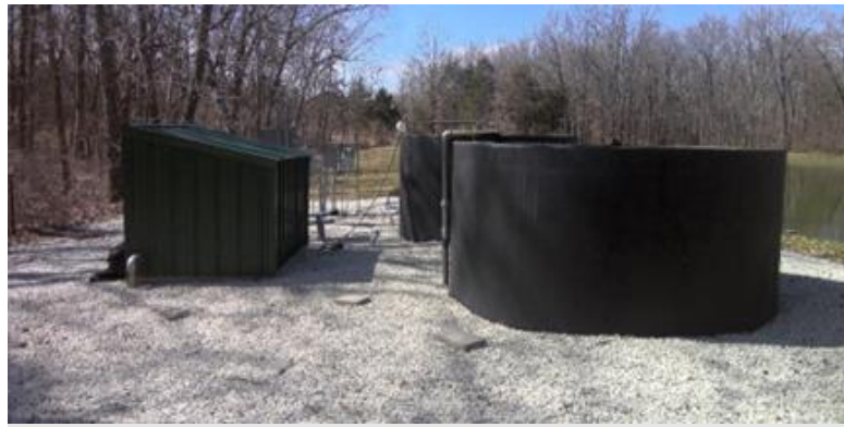
MBBR system added to Roy-L lagoon
