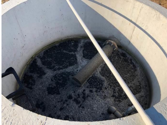
Example of side-stream MBBR at Twin Oaks Recirculating Sand Filter
