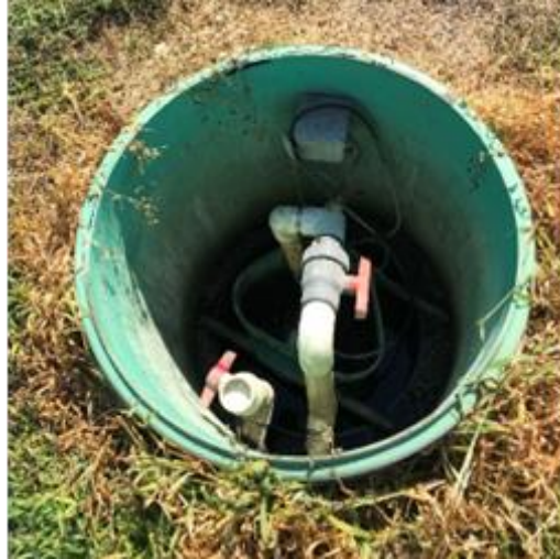
3 4 Failed distribution pump at Berkshire Glenn
