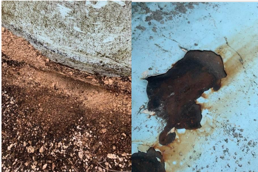
3 Erosion around standpipe gravel footing / corrosion to standpipe coating
