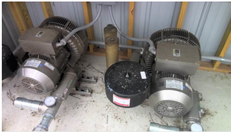
New blowers at the Chelsea Rose facility which had no functional blowers at acquisition
