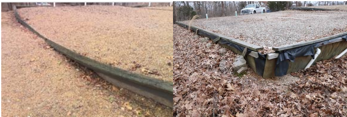
14 15 Bowed plywood wall and failing corners at Cimarron Bay Sand filter 16 17
