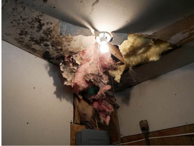
Failing insulation at Fawn Lake Well house, damaged interior
