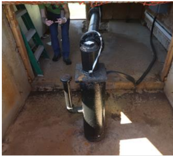
Rust on Well #3 well head.
