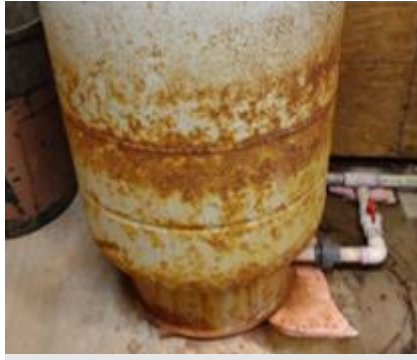
Rusting bladder tank at Missing Well system
