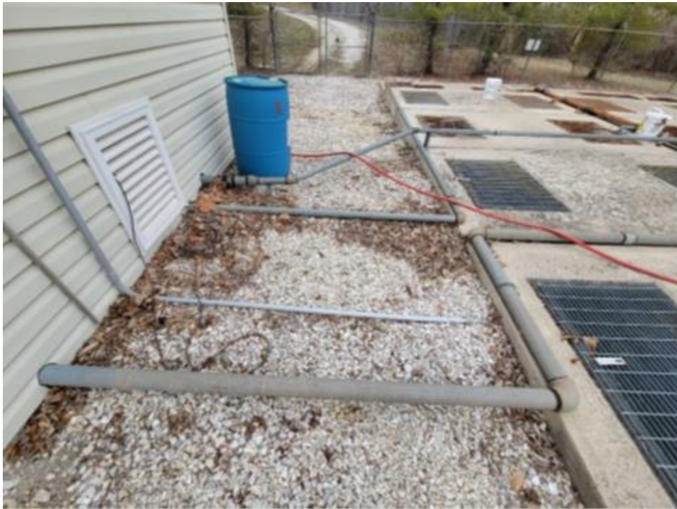
7 8 Undersized air headers causing issues with DO levels in portions of the aeration basins (3" piping to 9 aeration basins / 1.5" piping to the flow equalization basins)
