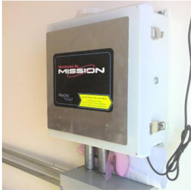
Remote monitoring system at Prairie Fields
