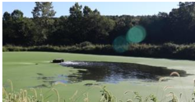
11 12 Underperforming surface aerator at Terre du Lac three-cell lagoon 13 14
