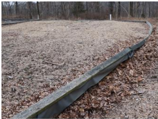
14 15 Vegetation debris on surface of Cimarron Bay filter beds.
