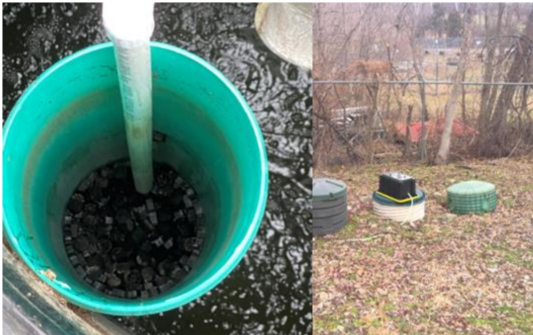
Drop in Micro MBBR and small blower at Cedar Glen facility.
