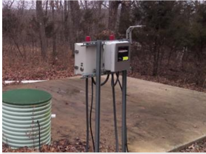
6 7 Remote monitoring unit at treatment facility
