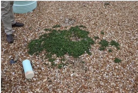
12 13 Vegetation growing on surface of Cedar Glen filter beds.
