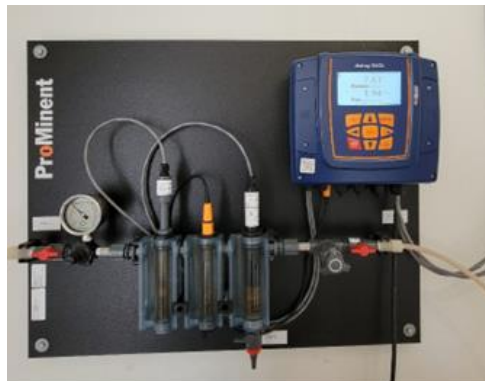
Chlorine Analyzer system (well #4)
