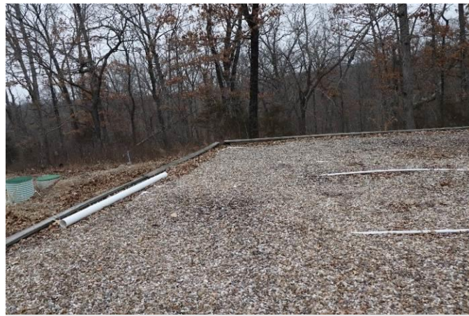
13 14 Exposed piping in Cimarron Bay filter beds
