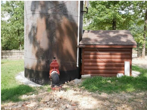
11 12 Significant rust at base of Branson Cedars standpipe tank
