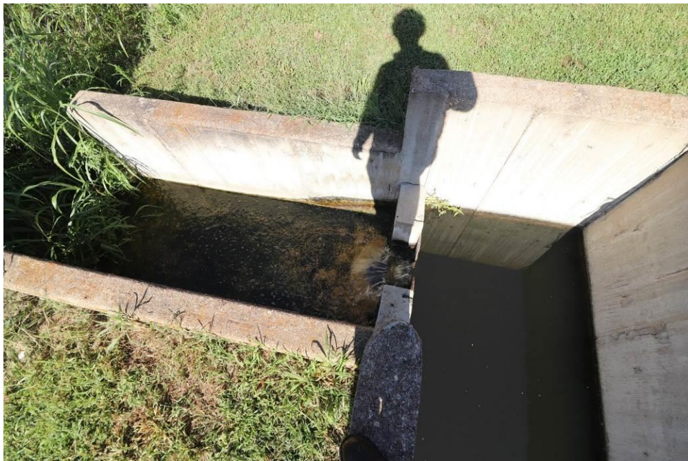
Dechlorination not installed at Terre du Lac Oxidation ditch
