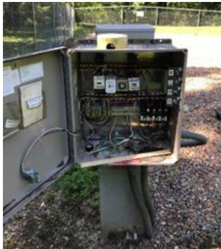
5 6 7 Failed power and control system at Fox Run
