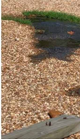
Sludge accumulation causing ponding on Cimarron Bay sand filter bed
