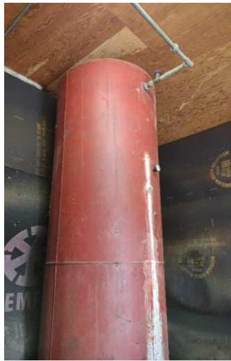
Leaking hydropneumatic tank in Well #1 well house
