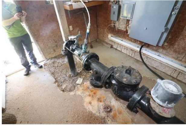
Well # 3 well house interior with damaged floor
