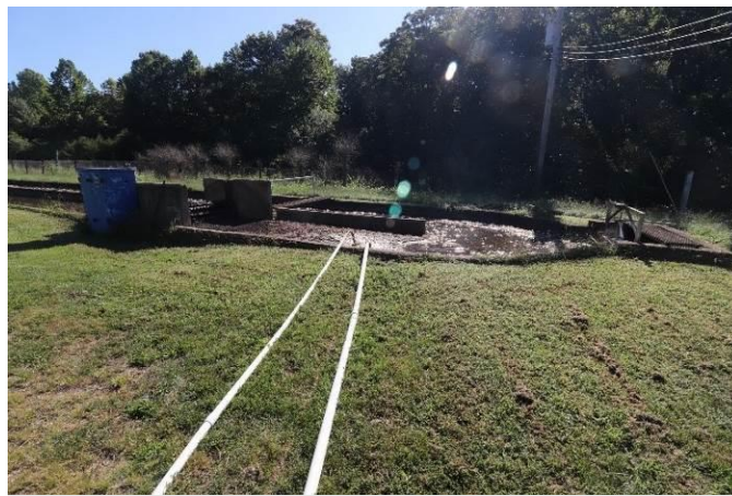
Above ground RAS lines at Oxidation Ditch
