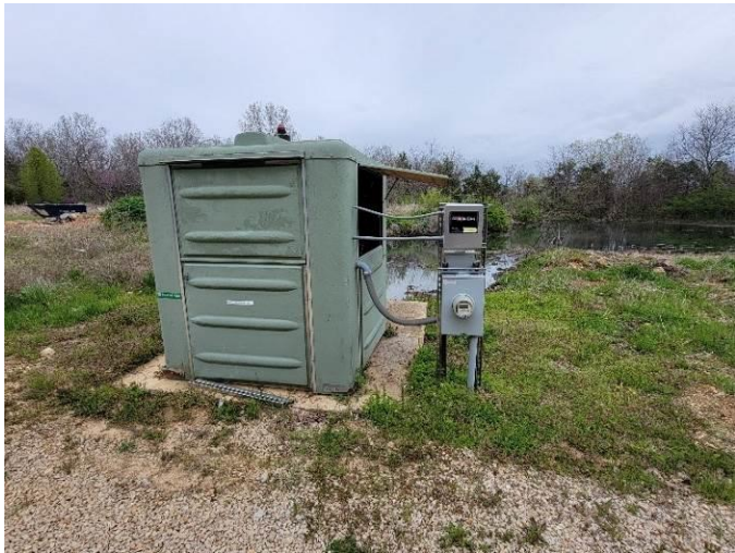
Example of Terre du Lac lift station with unapproved surge basin
