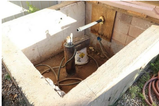
12 13 Inactive Well #1: exposed wiring and physical disconnection 14
