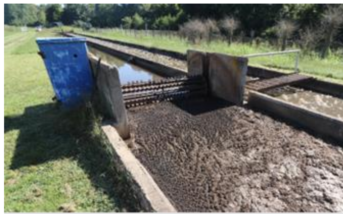
15 16 Failed brush aerator at Oxidation Ditch
