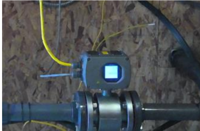
4 5 Magnetic Flow Meter at Cedar Glen Drinking Water system 6
