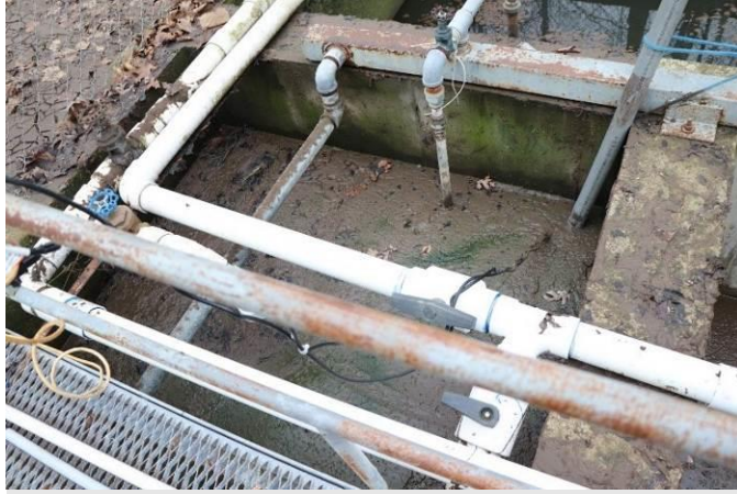
Rusting aeration piping partially replaced with PVC at Chelsea Rose, no functioning aeration and degraded diffusers present.
