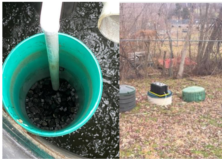
8 9 Micro MBBR in Recirculation tank and small blower running MBBR
