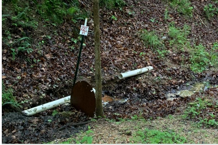
Outfall pipe terminating short of the receiving waters
