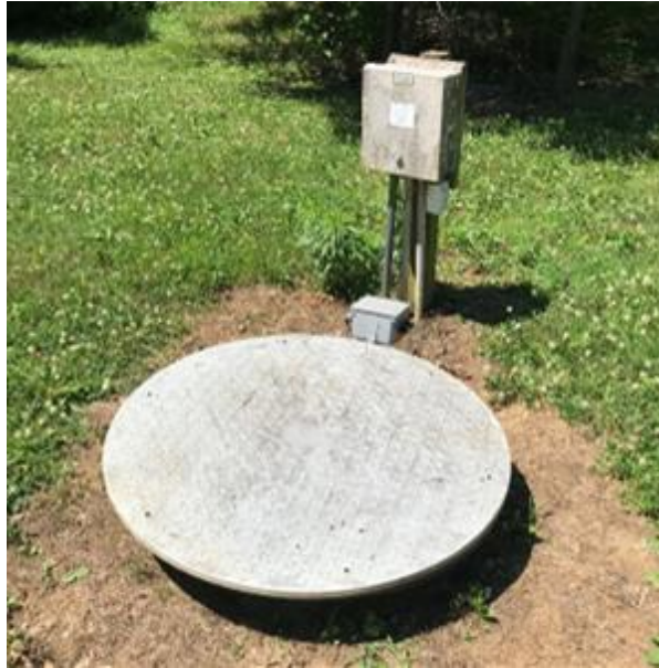
Lift station at Park Estates, missing redundant pump
