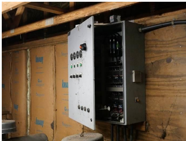
Damaged control system at Cedar Green facility
