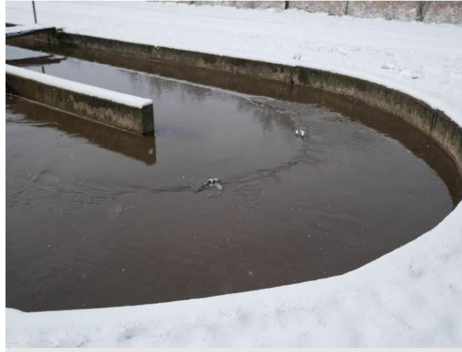
4 5 Sludge accumulation breaking the surface of water in the Oxidation Ditch
