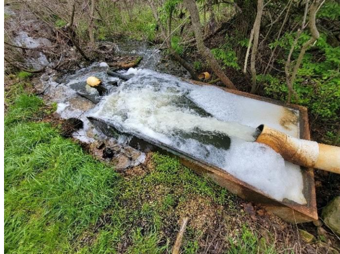
Disinfection system overwhelmed with high flows due to I&I issues. Note overflows over the sides of the contact chamber walls
