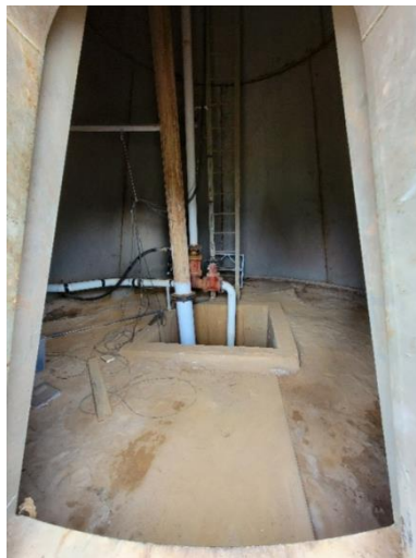
Interior tank near well #4
