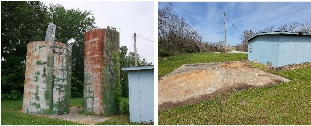
13 14 Deteriorating abandoned storage tanks at Fawn Lake (removed by Confluence Rivers)
