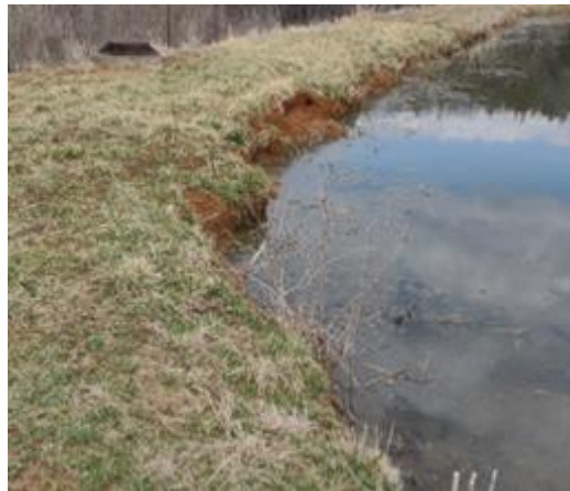
Varmint damage at Terre du Lac three-cell lagoon
