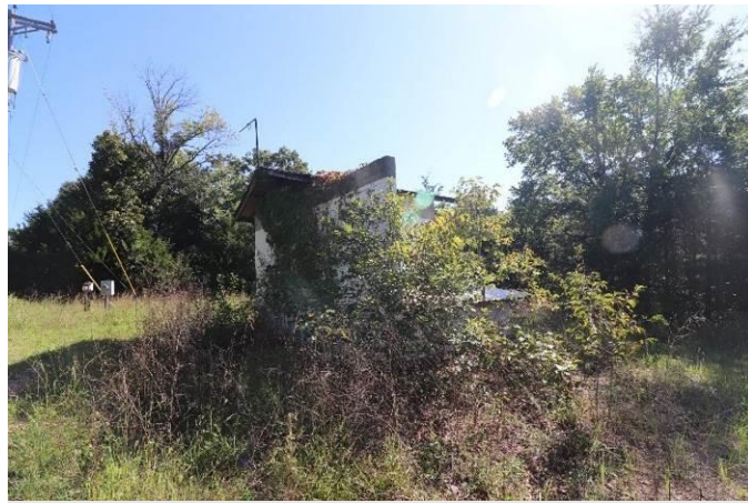
Vegetation overgrowing the Well #2 well house.
