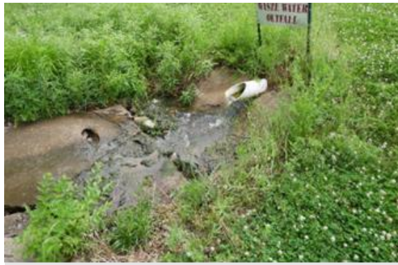
No disinfection present at Freeman Hills
