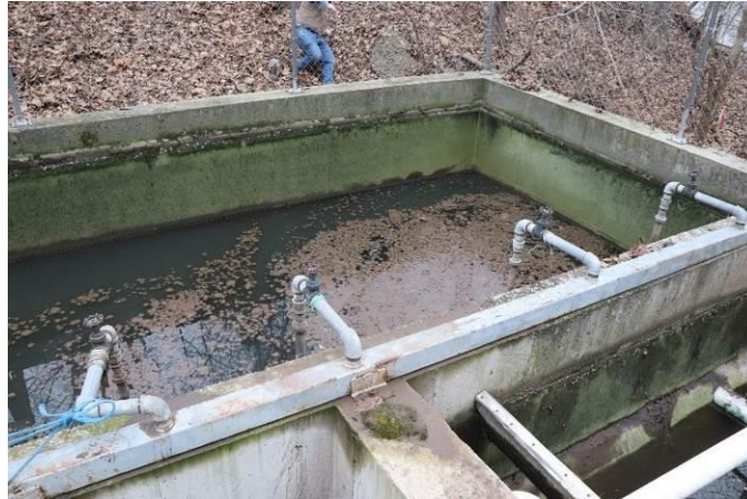
4 Poor condition of steel aeration piping (note blue ropes holding pipes in place at left) also note aeration 5 system was not running and floating sludge in aeration basin 6 7
