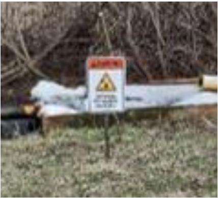
Overwhelmed disinfection system at Terre du Lac three-cell lagoon
