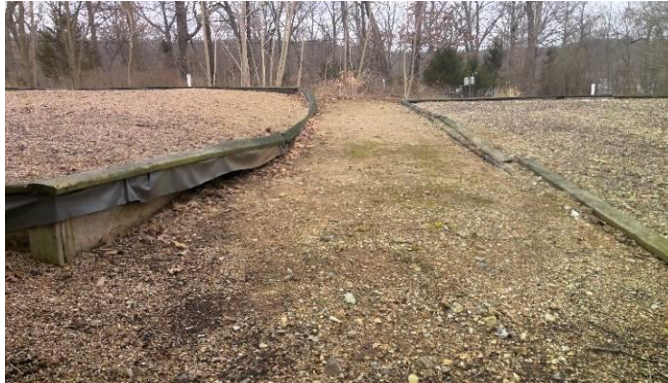
4 5 Failing wood structure at Cimarron Bay
