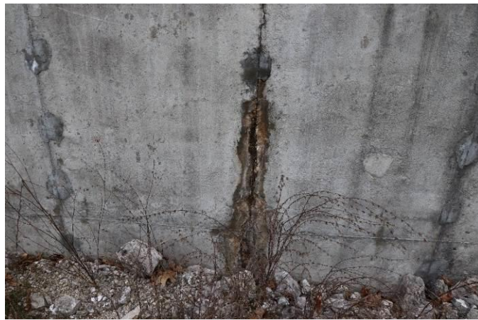
Cracks in concrete tankage
