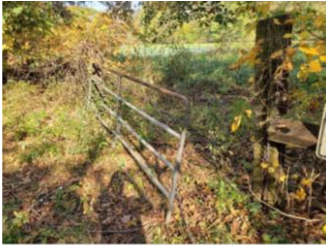
Fence damage due to overgrowth at Shelton Estates
