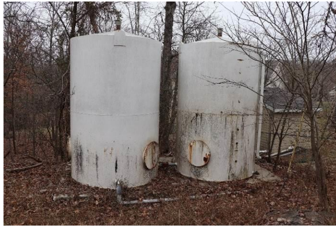
12 Condition of ground storage tanks at acquisition
