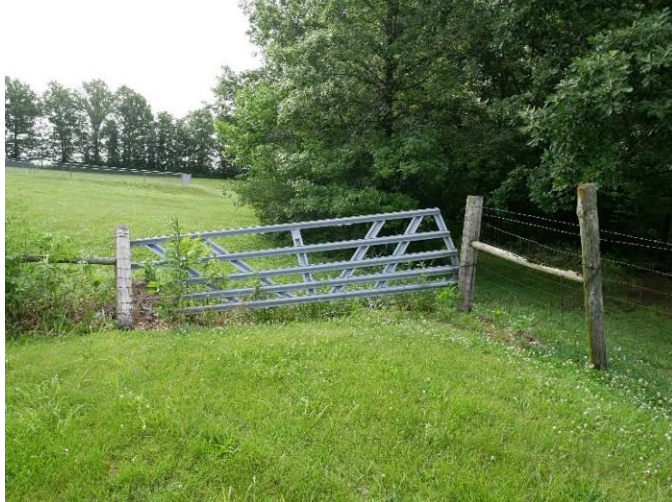
Examples of fence damage in need of repair
