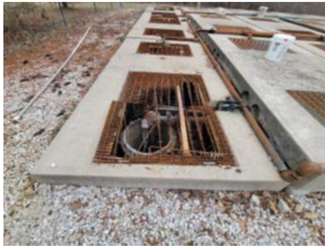
3 4 Rusted grating over the flow equalization tank.
