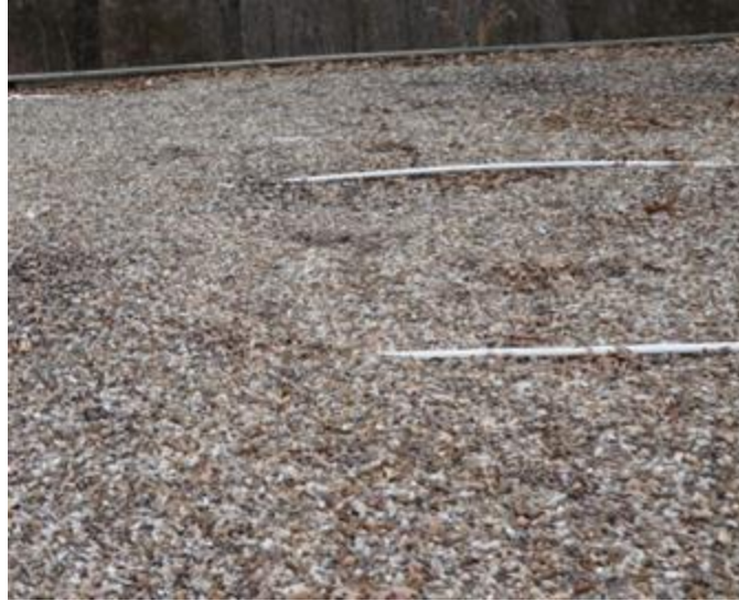
Damaged distribution piping at Cimarron Bay
