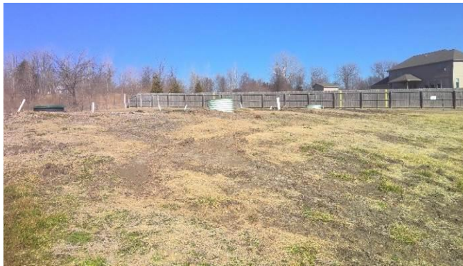
6 7 Evidence of leaks in earthen face of sand filter at Berkshire Glenn
