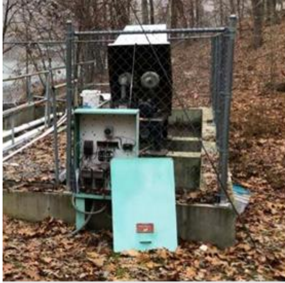
Poor condition/nonfunctional blowers and control system
