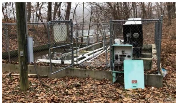
Failed control and power systems at Chelsea Rose facility
