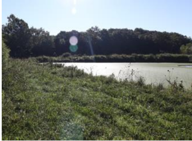
Poor condition of road around facility berm
