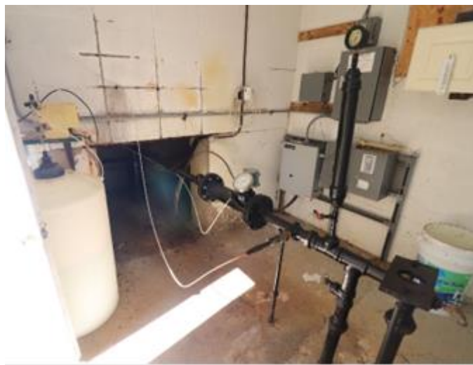
Interior of Well #2 well house.
