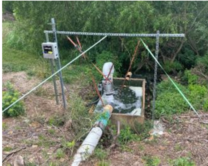
3 4 Temporary installation of flow meter and remote monitoring, note that while flow is still excessively high it 5 is significantly reduced from flow at acquisition 6
