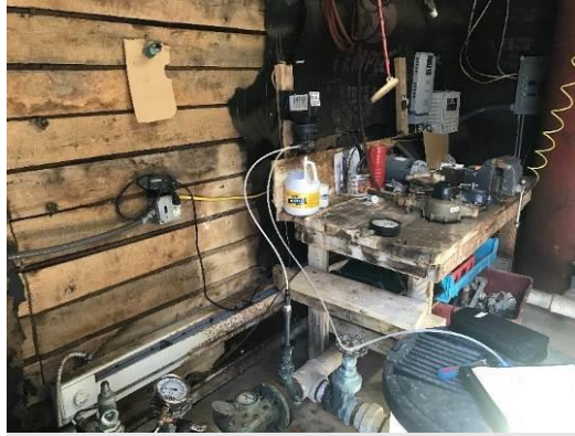
Housekeeping and electrical issues in Well #1 well house
