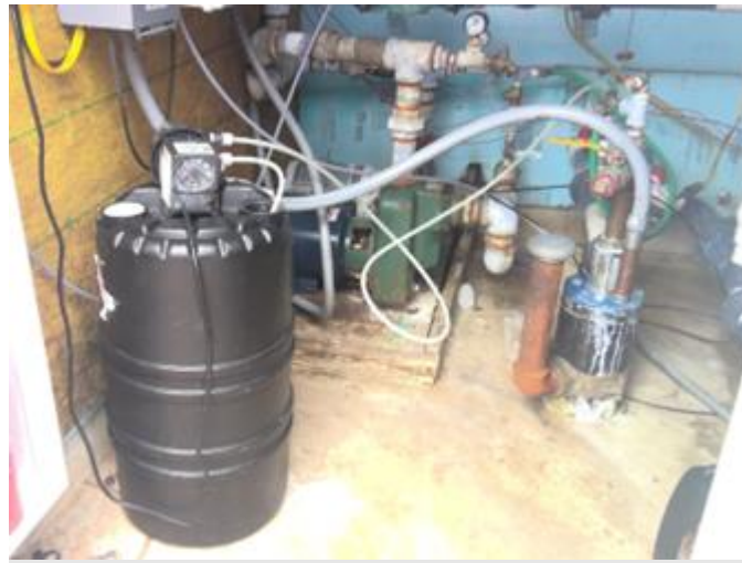
New disinfection system, improved wiring, piping, etc.
