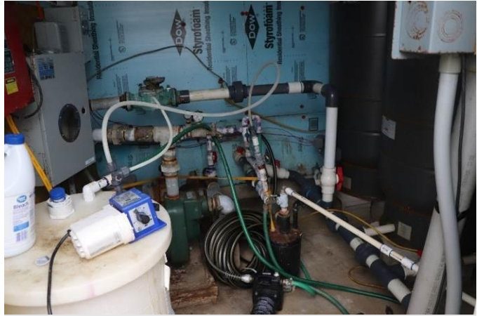
4 Well house interior, note coils of garden hose, rusted well head plate, exposed wiring, bleach bottle
