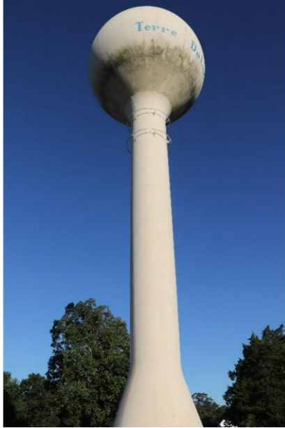
Tank near well #1
