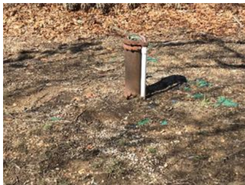
Rust and improper electrical wiring at Well #1 well head
