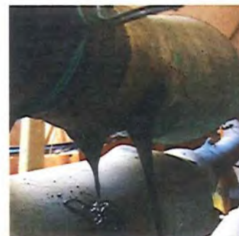
Abnormal PILC cable joints
