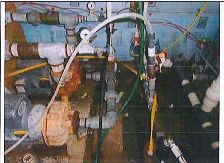
Location: Eagle Woods Subdivision Photographer: Darrell Barber Photograph Date: June 11, 2014 Comments: Booster pumps (5-hp) and related piping.
