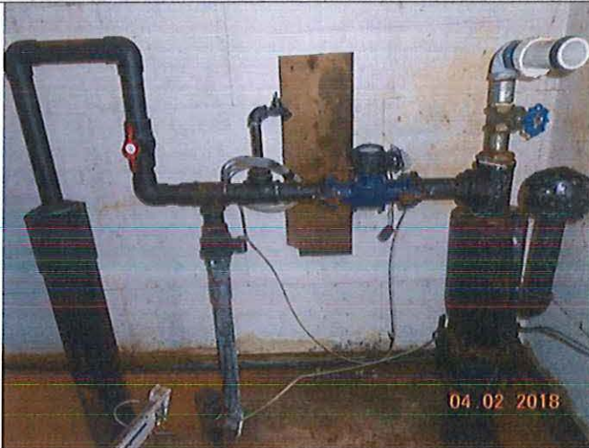
PHOTOGRAPH #1 TAKEN BY: Sheila Yoder ENTITY: Chelsea Rose Subd PERMIT: MO3031244 LOCATION: wellhouse DESCRIPTION: well #2 DATE TAKEN: April 2, 2018 PROGRAM: Public Drinking Water Branch
