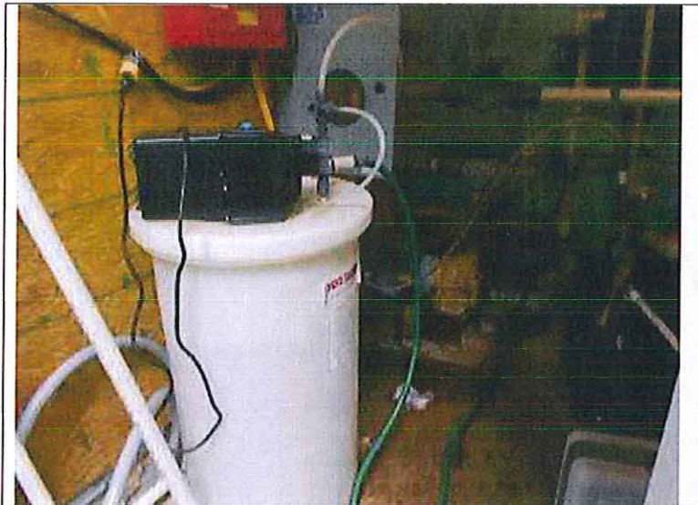
Location: Eagle Woods Subdivision Photographer: Darrell Barber Photograph Date: June 11, 2014 Comments: Chem-Tech (Series 200) chemical feed pump, 25-gallon chlorine solution tank and related piping.
