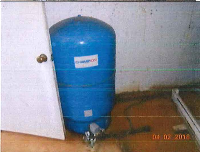
PHOTOGRAPH #2 TAKEN BY: Sheila Yoder ENTITY: Chelsea Rose Subd PERMIT: MO3031244 LOCATION: wellhouse for well#2 DESCRIPTION: bladder tank DATE TAKEN: April 2, 2018 PROGRAM: Public Drinking Water Branch
