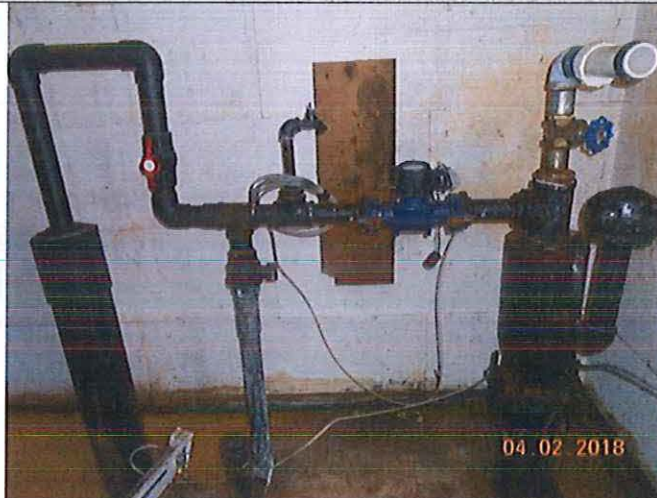
PHOTOGRAPH #1 TAKEN BY: Sheila Yoder ENTITY: Chelsea Rose Subd PERMIT: MO3031244 LOCATION: wellhouse DESCRIPTION: well #2 DATE TAKEN: April 2, 2018 PROGRAM: Public Drinking Water Branch
