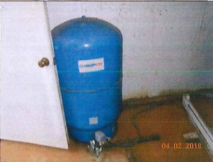
PHOTOGRAPH #2 TAKEN BY: Sheila Yoder ENTITY: Chelsea Rose Subd PERMIT: MO3031244 LOCATION: wellhouse for well#2 DESCRIPTION: bladder tank DATE TAKEN: April 2, 2018 PROGRAM: Public Drinking Water Branch
