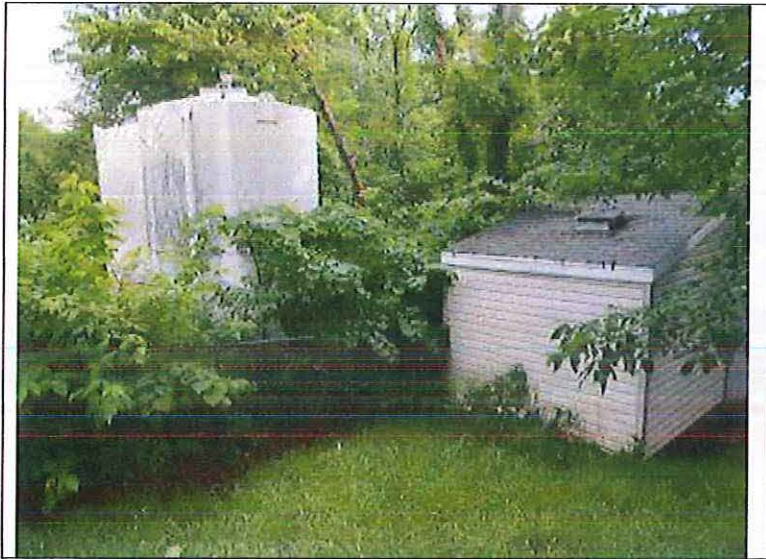
Location: Eagle Woods Subdivision Photographer: Darrell Barber Photograph Date: June 11, 2014 Comments: Well house and two 4,500-gallon ground storage tanks.
