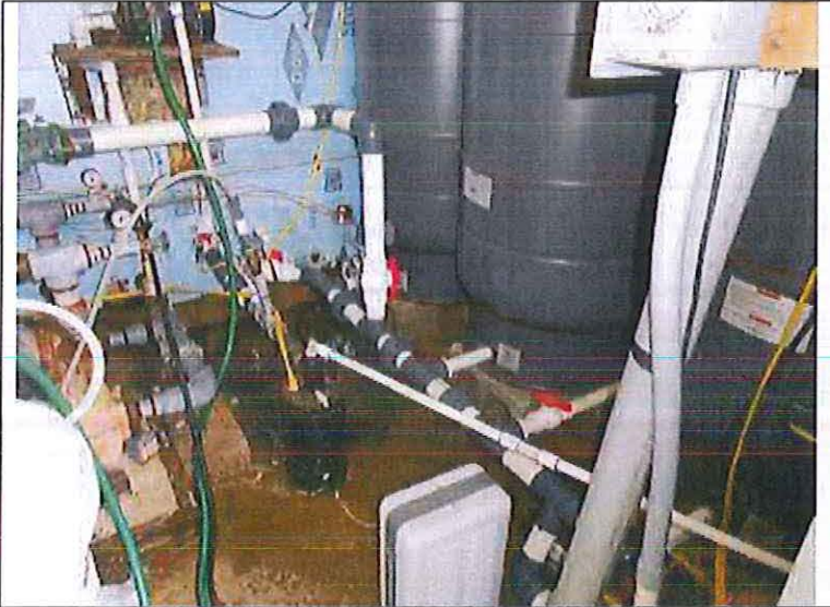
Location: Eagle Woods Subdivision Photographer: Darrell Barber Photograph Date: June 11, 2014 Comments: Well, three 119-gallon bladder tanks and related piping.
