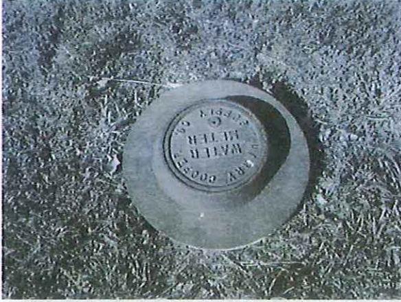
Riverfork Ranch—Typical meter vault cover
